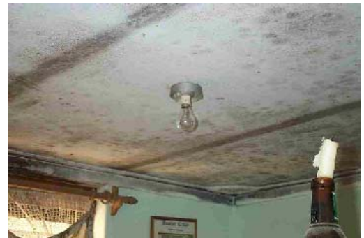
Mould growth on a ceiling
