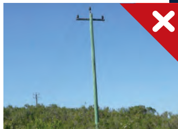
Non-compliant: thick scrub creates a fire hazard around power poles
