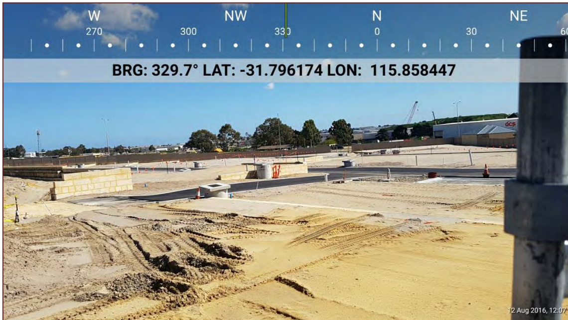
Plate 5: Excluded areas west of the project area consistent with Clause 2.2.3.2 (e) of AS 3959 2009
