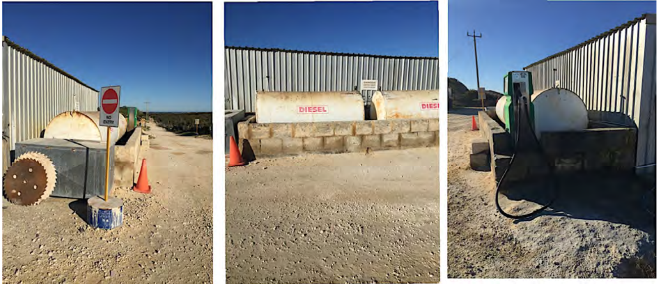
On site fuel tank
