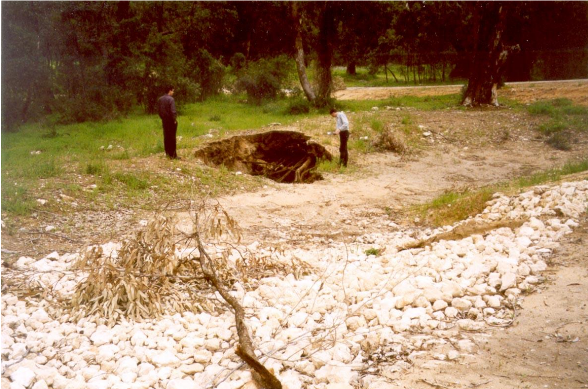
Figure 2 - Sinkhole within road drainage discharge area, Emerald Drive, Carabooda.
