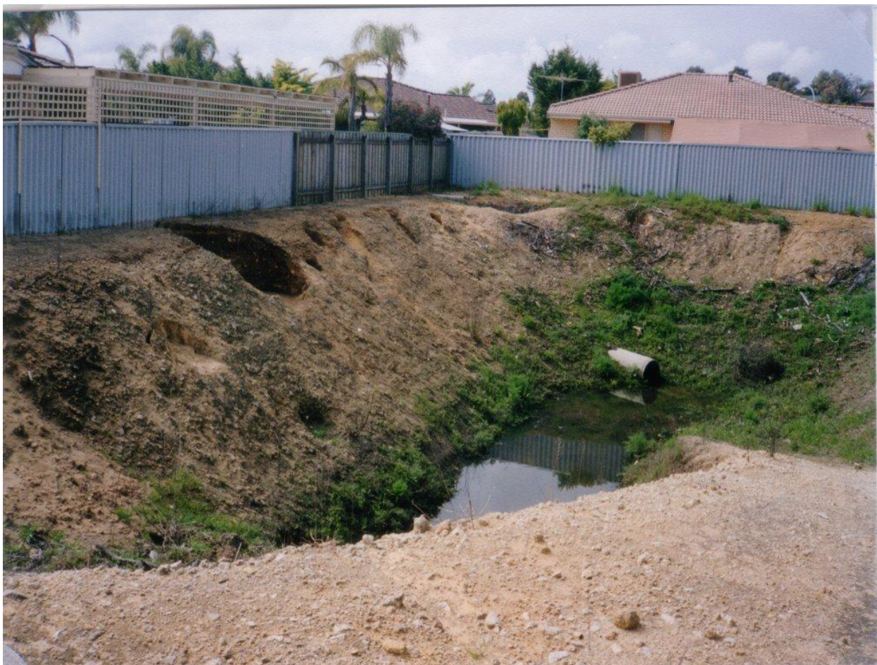
Figure 1 – Road drainage basin at Regatta Drive, Edgewater showing sinkholes on left and at rear.
