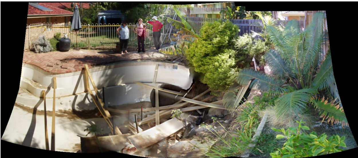
Figure 3 - Woodvale swimming pool with bracing following collapse
