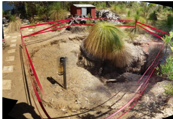
Figure 4b - Breakwater Drive, Two Rocks. Close up view of sinkhole. Note tension crack around edge of failure zone
