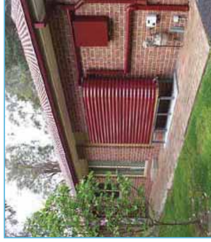
Slimline domestic rainwater tank
