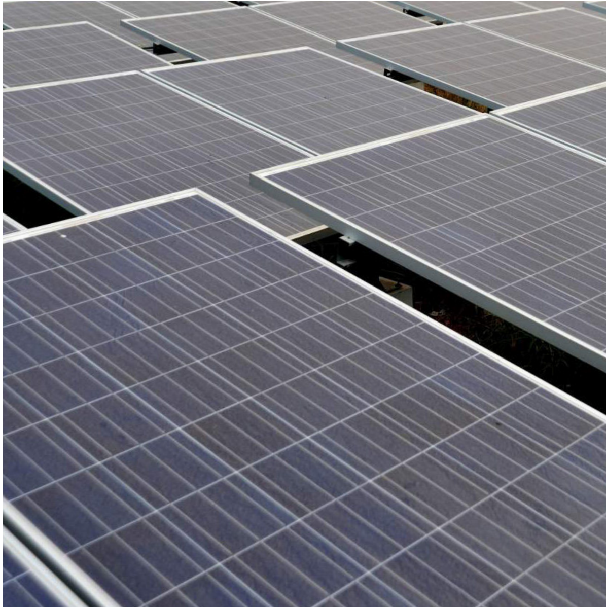
Solar Canopy / Array on Rooftop to maximise solar gain.
