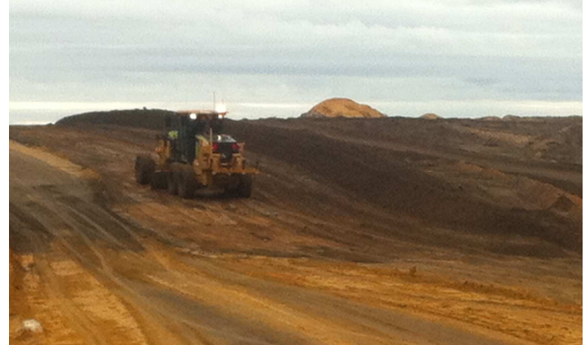
Earthworks underway on the eastern side of the train line near Burns Beach Road.
