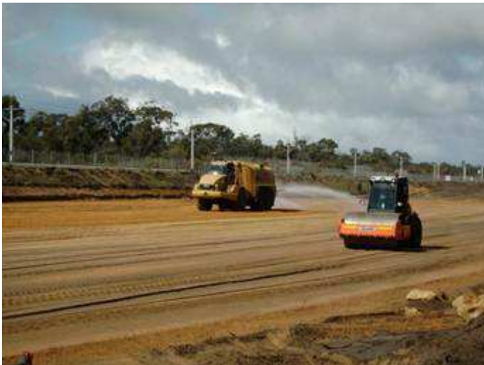
Water carts and rollers used to compact new material as the ground level is built up.
