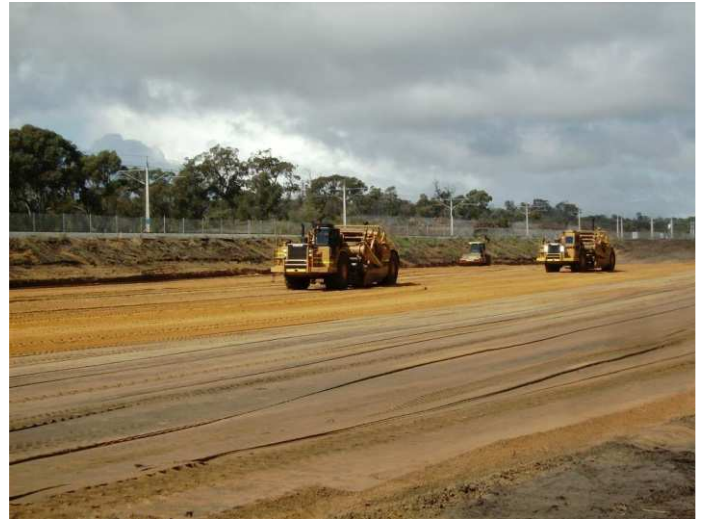
Scrapers used to move excess material near Clarkson Train Station further north to increase ground levels.
