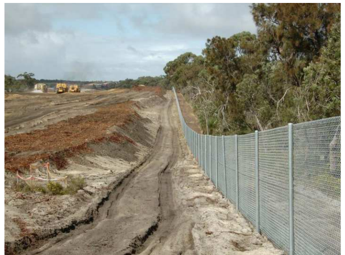
Permanent fencing installed along the boundaries of the road reserve, and between the train line and the freeway alignment.
