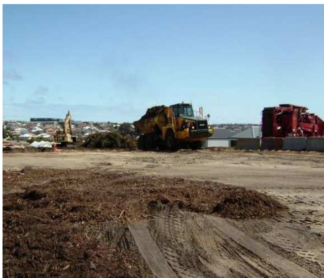
Removed vegetation is mulched and stockpiled within the worksite for re-use at the end of the project
