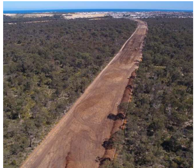
Aerial view of Neerabup Road extension looking west where earthworks are underway.
