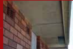
Unsecure eave joints
