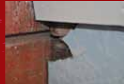
Damaged Tilux in bathrooms or laundries
