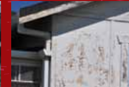
Exposed asbestos due to peeling paint
