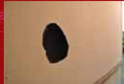
Holes in fibro walls
