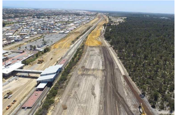
Aerial views of the freeway alignment looking south (top) and north (bottom) from Neerabup Road extension.
