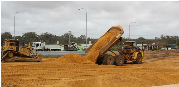
Material is being imported to build up the levels of the new Wanneroo Road carriageway.
