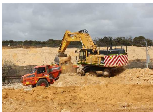
Excavator loading material into an Articulated Dump Truck near Kinross. These trucks can carry up to 40 tonnes of material per load.
