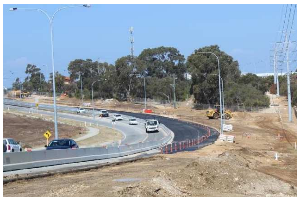
Hester Avenue traffic will soon be travelling on new section of road to the south.
