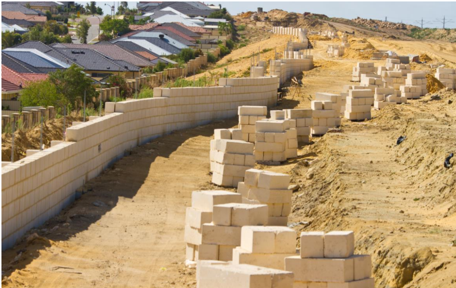
Above: Noise wall construction underway adjacent to the future Mitchell Freeway alignment.
