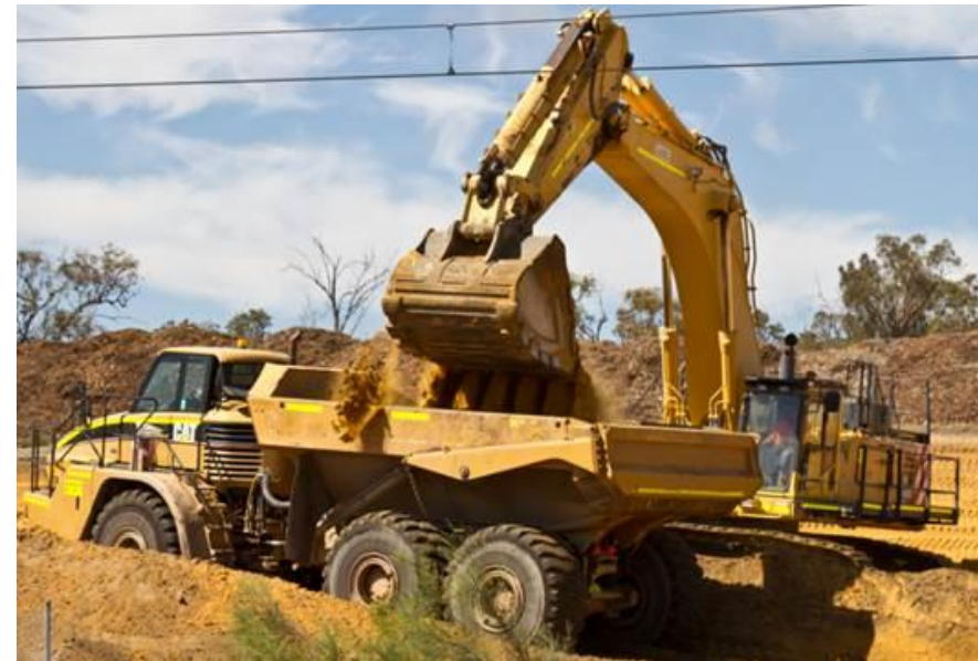
Above: Earthworks taking place as part of the extension of Neerabup Road to Wanneroo Road / Flynn Drive.
