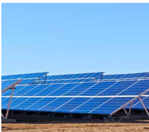
Solar Power Station
