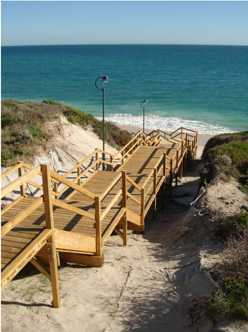
Plate 13 Example of boardwalk steps for one of the proposed beach access points.
