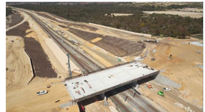
Above: Progress of construction of the new Mitchell Freeway/Neerabup Road interchange bridge
