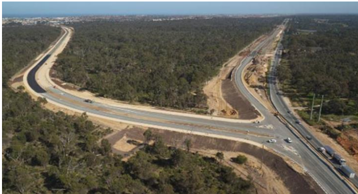
Above: Progress of construction of the new Wanneroo Road/Flynn Drive/Neerabup Road intersection
