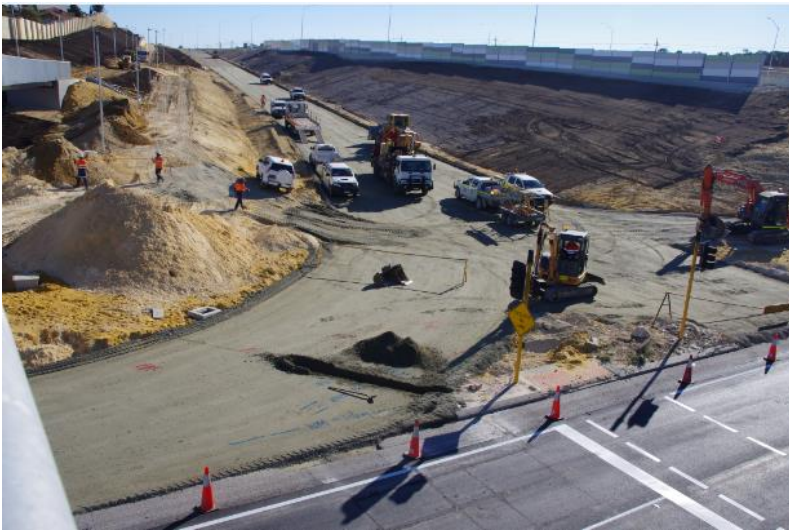
Above: Base-course works on the new Burns Beach Road on-ramp to Mitchell Freeway northbound
