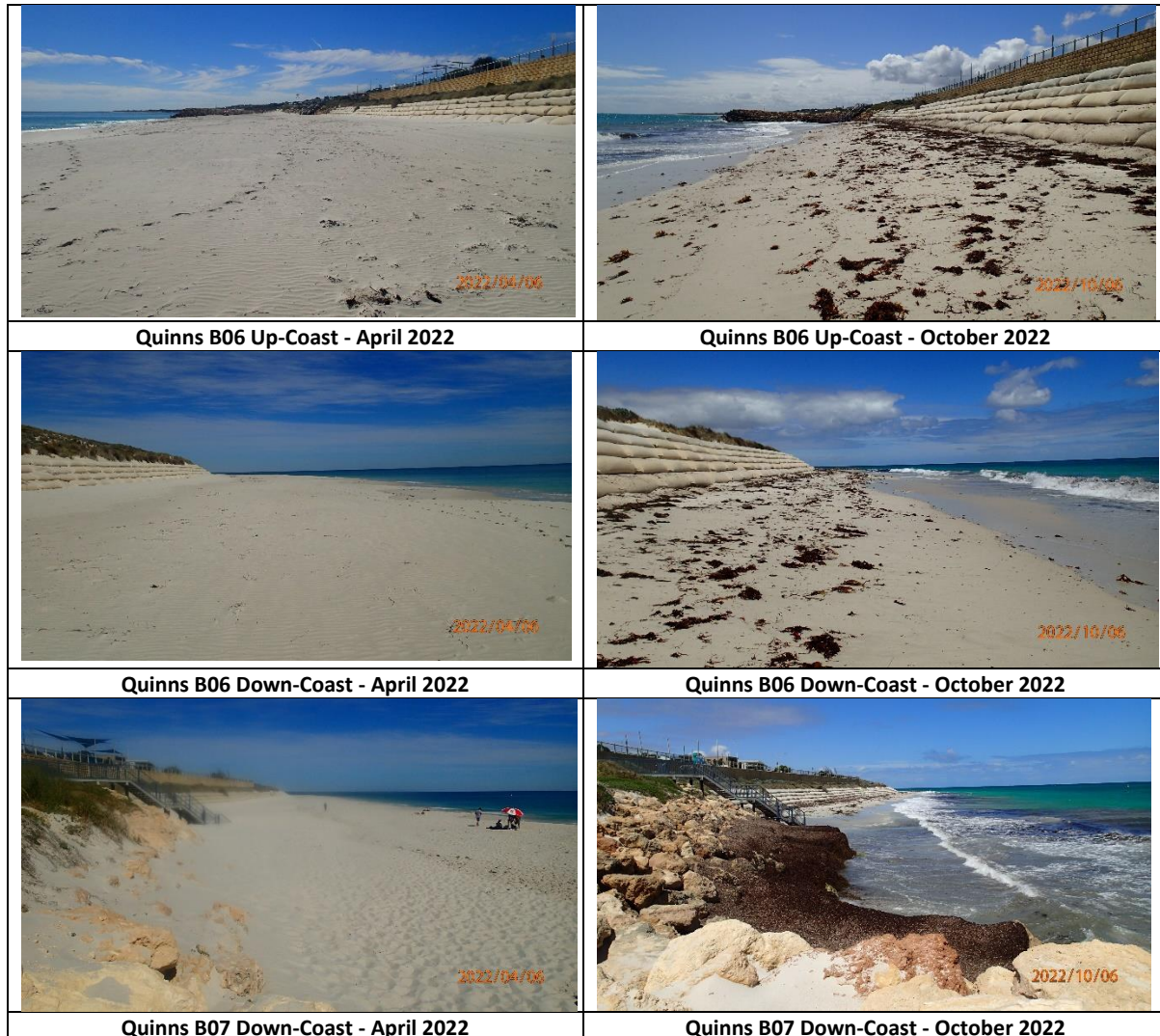
Figure 4-8 Major erosion over winter 2021 at Quinns B06 Up-Coast, Down-Coast and Quinns B07 Down-Coast.
