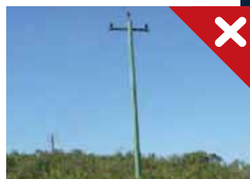
Non-compliant: thick scrub creates a fire hazard around power poles
