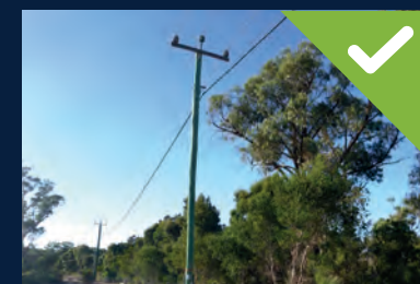
Compliant: cleared buffer zone around power poles
