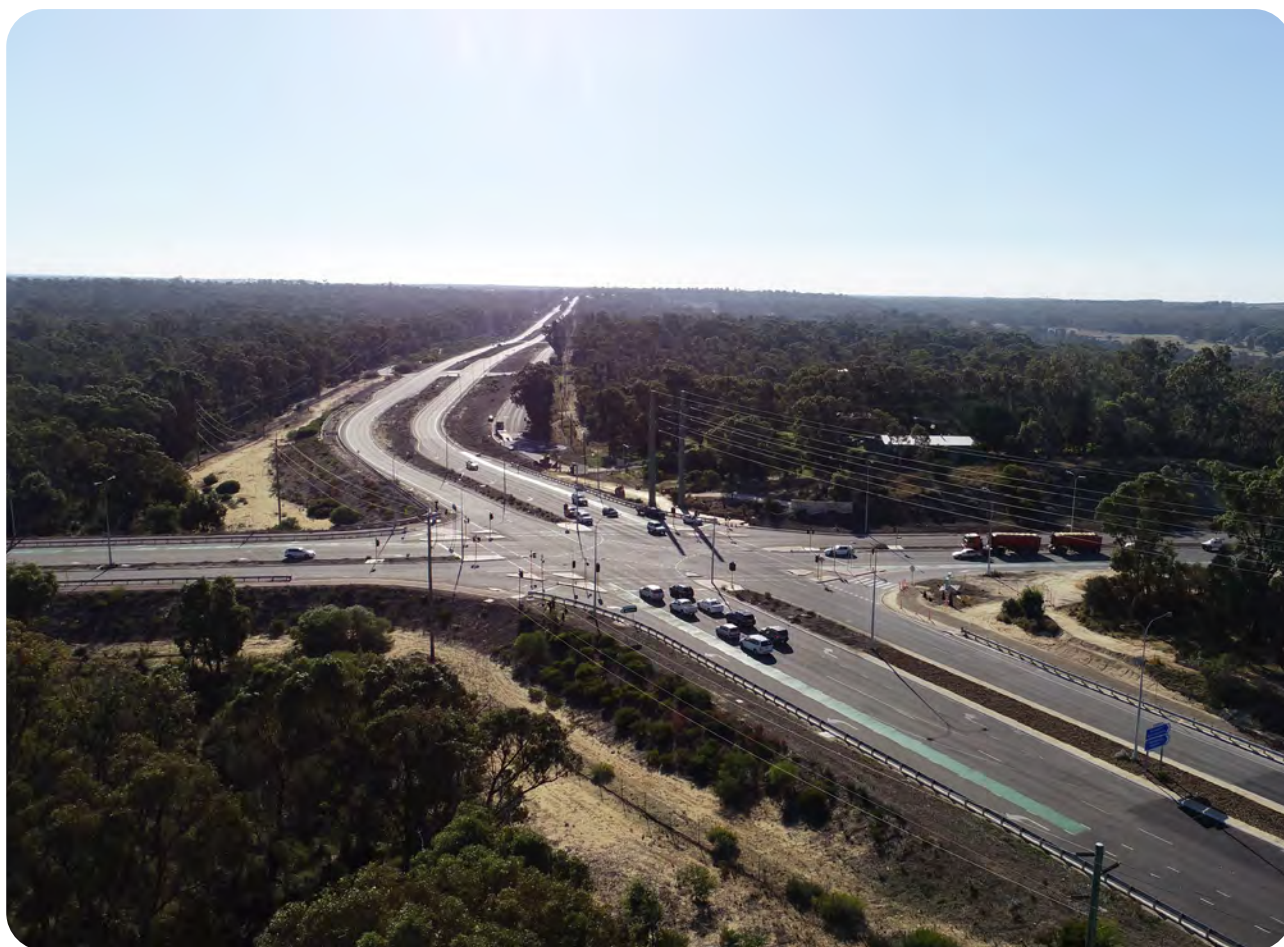
The upgrade of Flynn Drive will provide an important strategic transport link ▲ for the fast-growing industrial area at Neerabup. ▲
